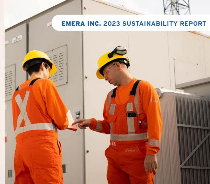
Nova Scotia Power team members at the Intelligent Feeder Battery Storage Pilot in Elmsdale, NS.
